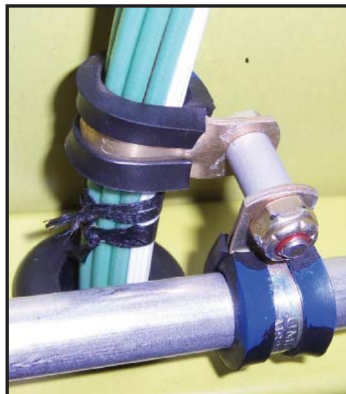
Figure 1-2: Left Main Wiring Harness and Wing Fuel Vent Line
